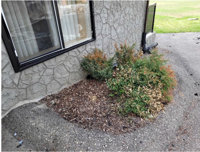
Figure 47: Mulch bed beneath window of structure with visible damage adjacent to the burned structures.
