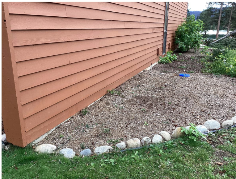
Figure 28: Vulnerability (mulch under combustible siding) that was also present on the burned structure on the shore of Beauvert Lake. Photo of identical adjacent unburned structure to show likely state before burning.
