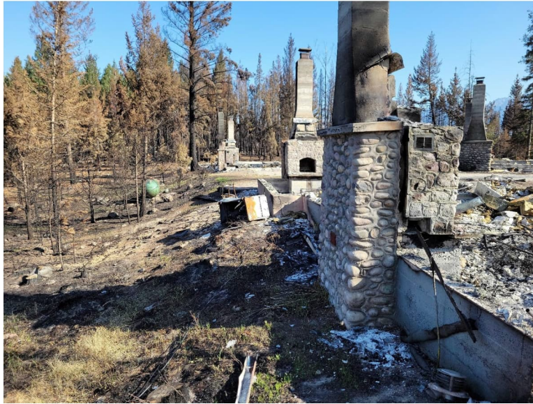
Figure 42: Continuity of wildland fuels on the west side of the burned structures in the northwest portion of Tekarra Lodge.
