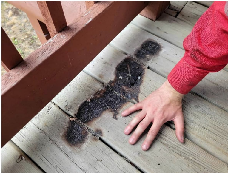
Figure 32: Burning of a surviving structures deck in Thornton Village. Ignition likely started from an ember in the tight crack between the ends of the deck boards where the most mass loss has taken place.
