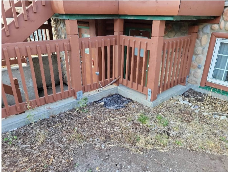
Figure 31: Ignited organic matter buildup around a surviving structure in Thornton Village.
