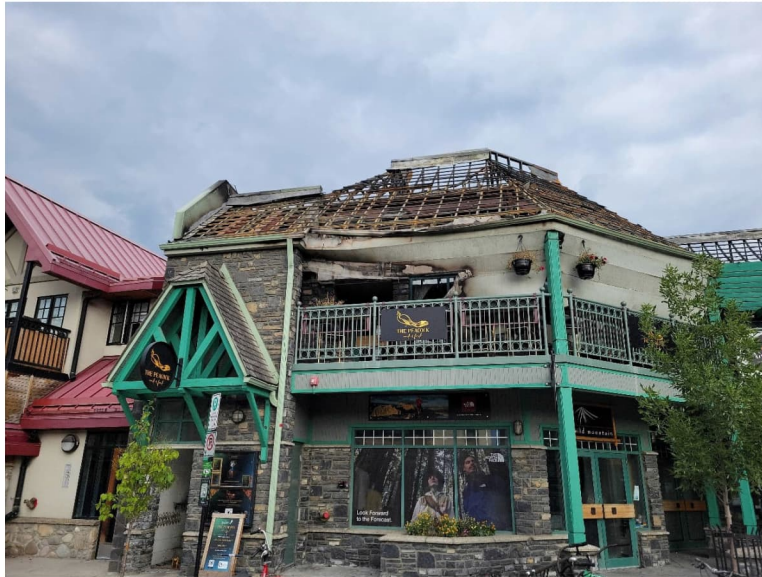
Figure 19: Wood shake roofing ignited by embers in the commercial area of Jasper townsite.
