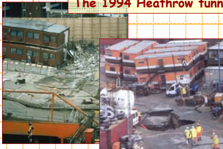
The 1994 Heathrow tunnel collapse.
