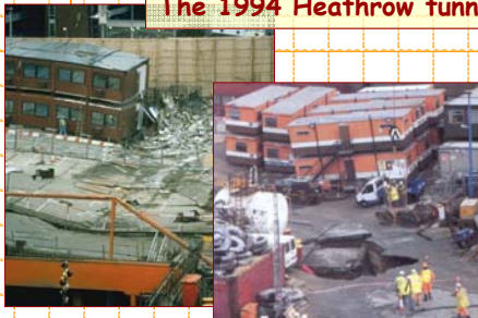
The 1994 Heathrow tunnel collapse.
