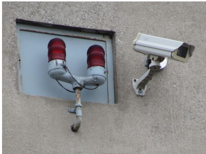
Fig. 17 A photograph of the aircraft warning lights and security camera as mounted on the side of the York University Stack
